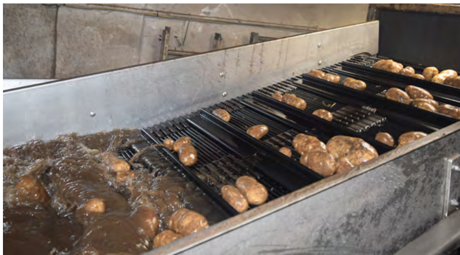
The Kitchen Kleen Russet Burbank potatoes are washed before being conveyed from a warehouse to the new packing shed at Nuto Farm Supply.
