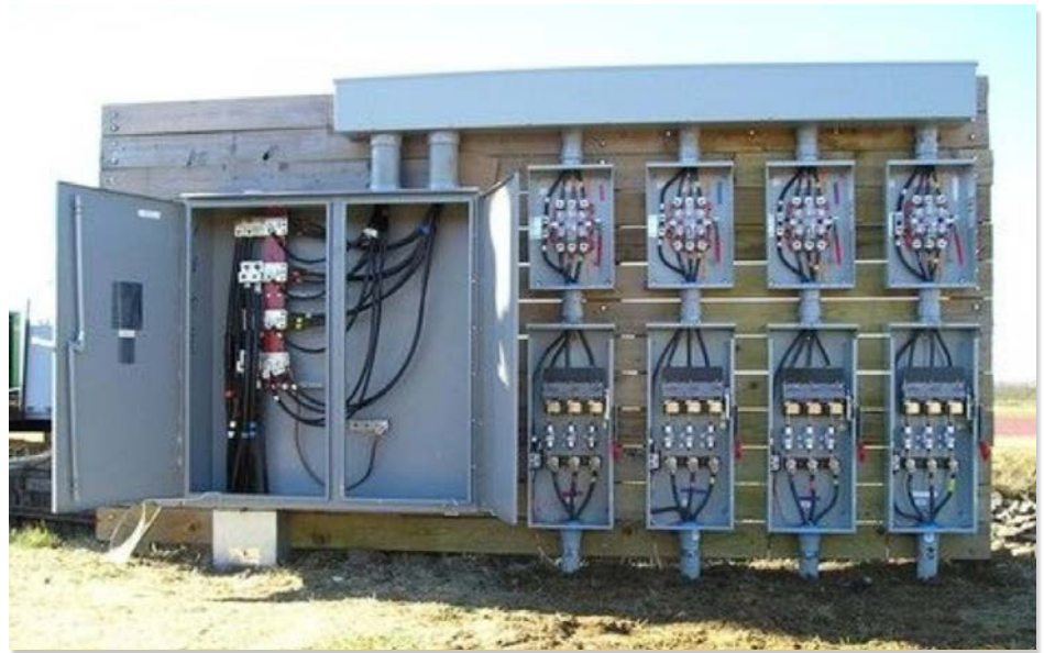
An electrical control panel is set up and ready for use at a local farm site.
